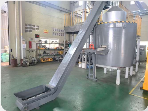
Continuous Casting Furnace (2t/Chg.)
